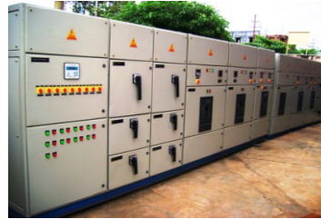
Power Distribution Panel
