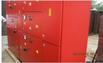
Fire Fighting Panel
